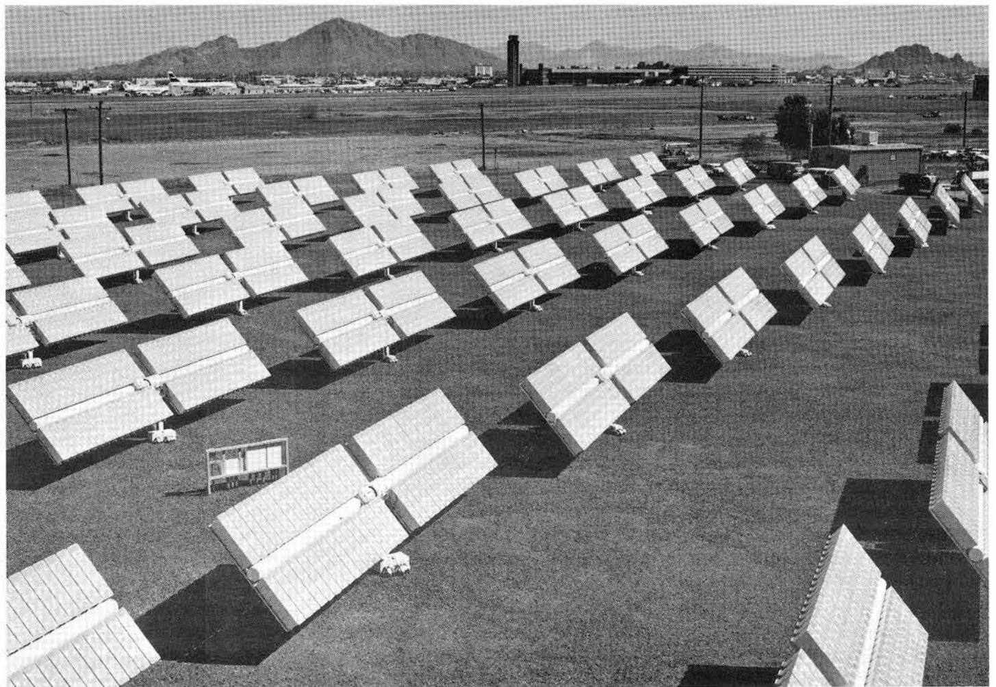
WORLD'S MOST EFFICIENT large-scale photovoltaic system, based on a design originated by Sandia, produces more than 230 kW peak output. It was developed by Mar-
